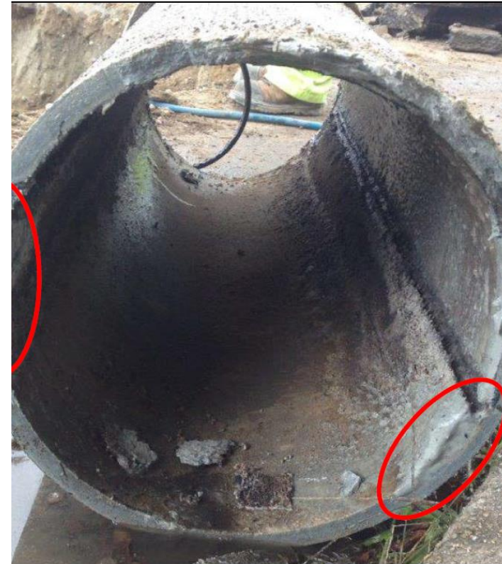
Delaminated areas of AC pipe
